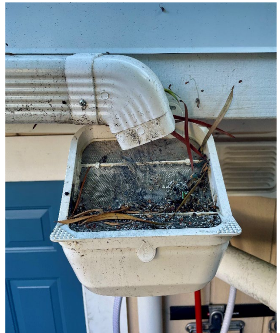
Example of a typical leaf filter. Note common debris that can accumulate from a roof including leaves, dead insects, and roofing particles. Debris should be cleaned off prior to rain.
